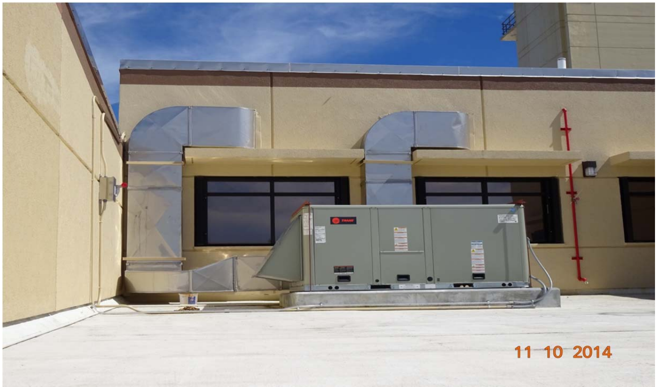
PACKAGE COOLING UNIT ( PCU)
