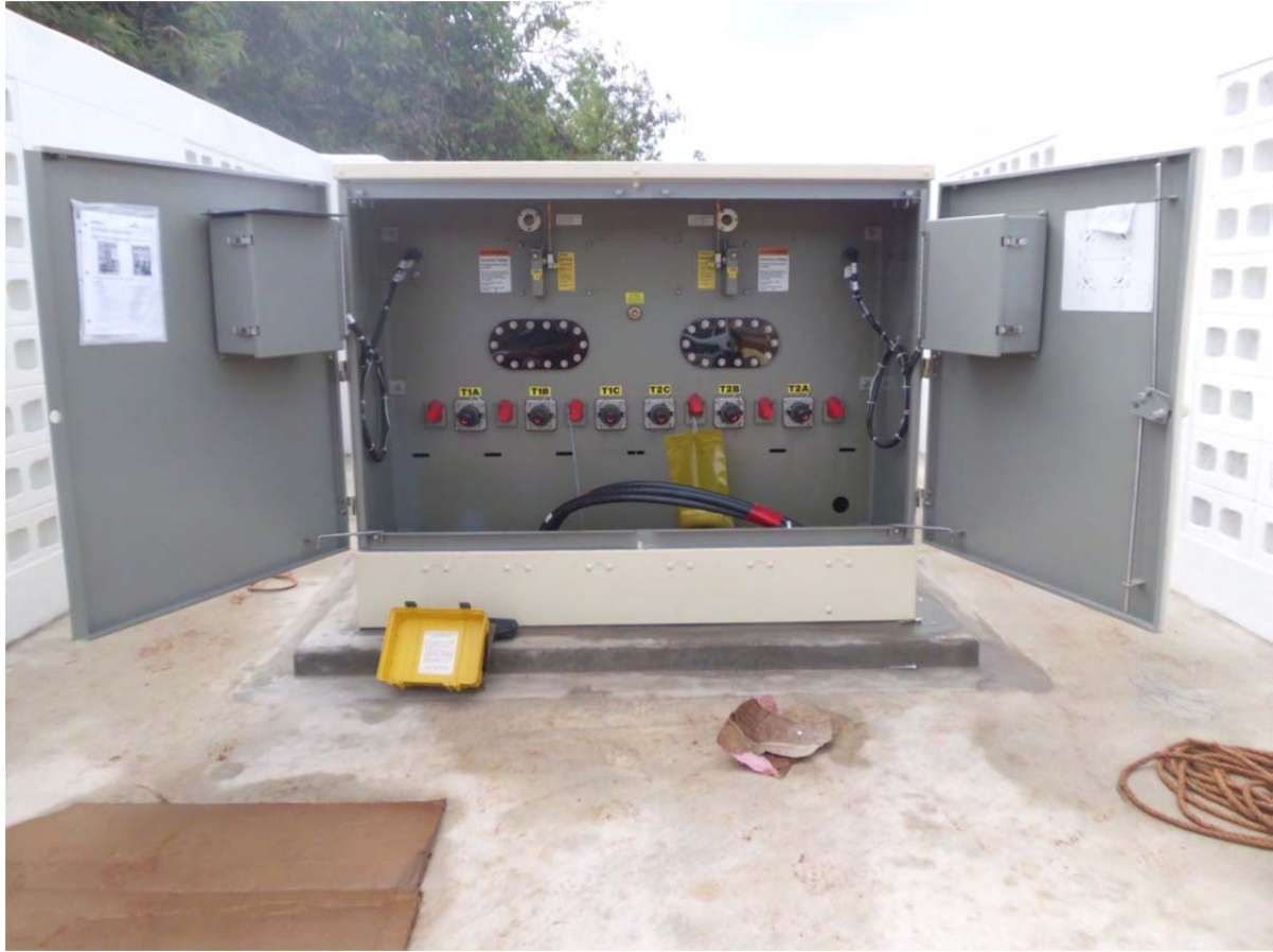
4-WAY PAD-MOUNTED SWITCHGEAR
