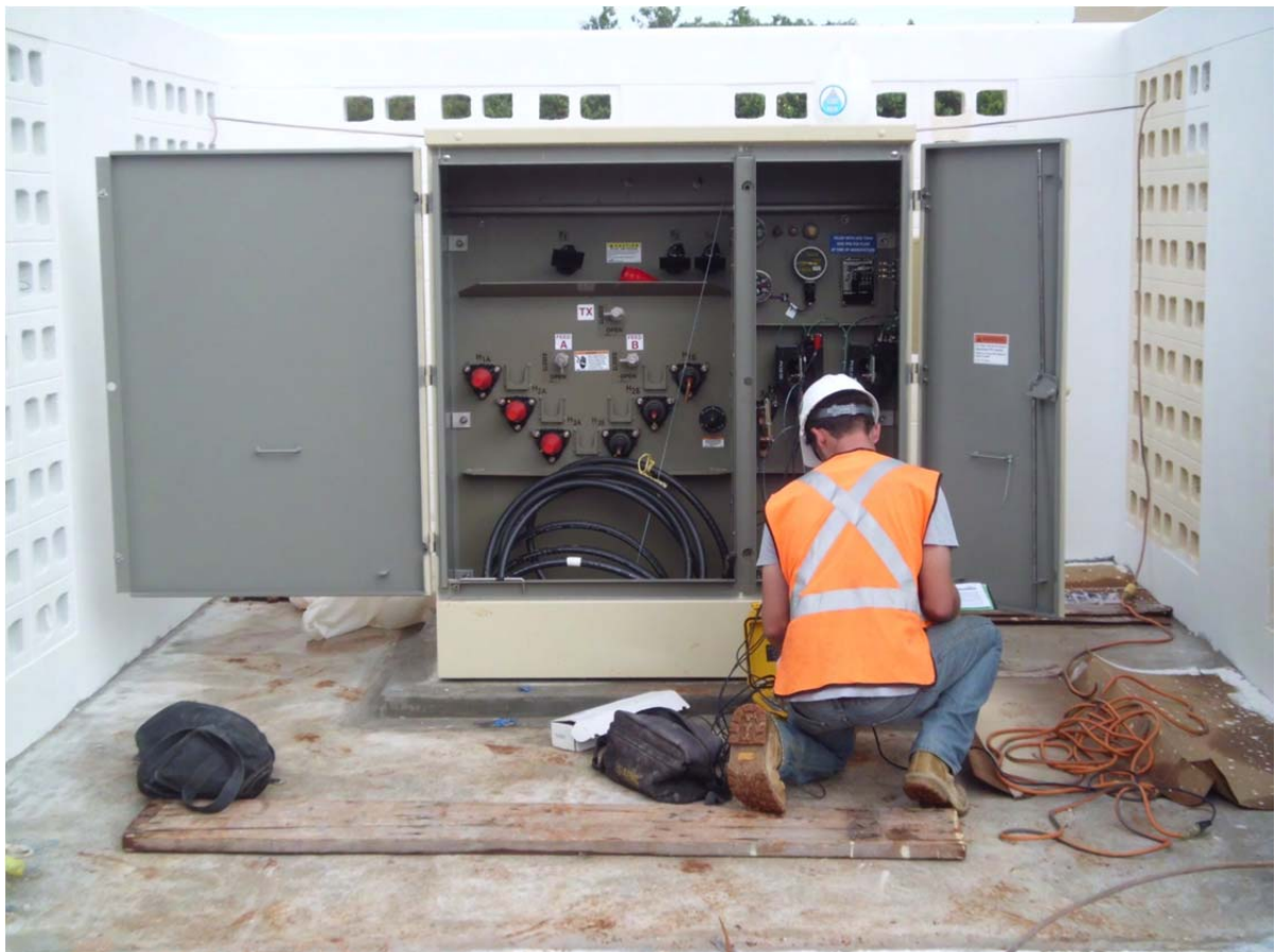
75 KVA PAD-MOUNTED TRANSFORMER
